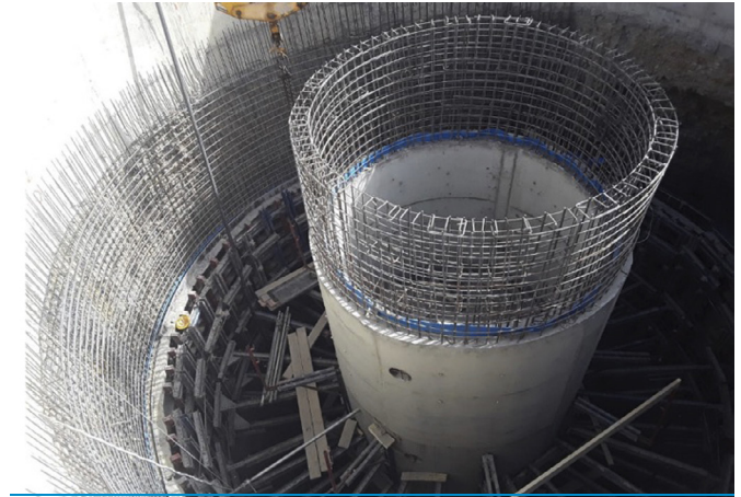
Figure 5 | A 4 m -diameter drainage well of the Hay Sadri neighborhood stormwater tunnel, part of the SRE system in eastern Casablanca.
