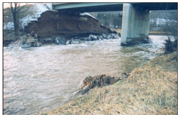
Figure 2. Failure of earthfill embankment at abutment
