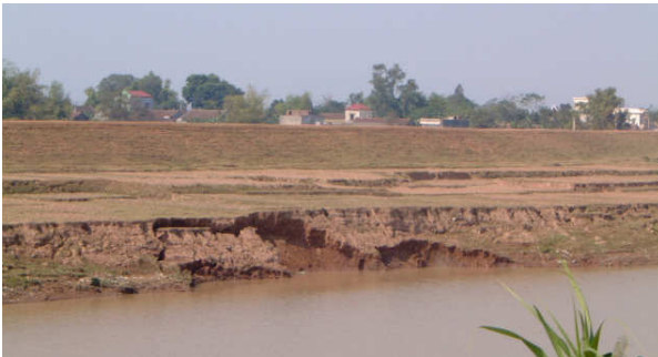
Figure 13. Example of a sliding due to toe scour in an outer bend
