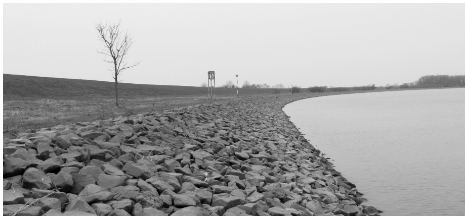
Figure 1. Rip-rap on the banks of Ems River (Germany) as a protective layer to prevent erosion of bank slope by hydraulic loads.
