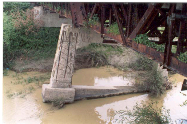
Photo nr. 4. Mifoli bridge. It's looking to north, and shows, the sinking of its pier
