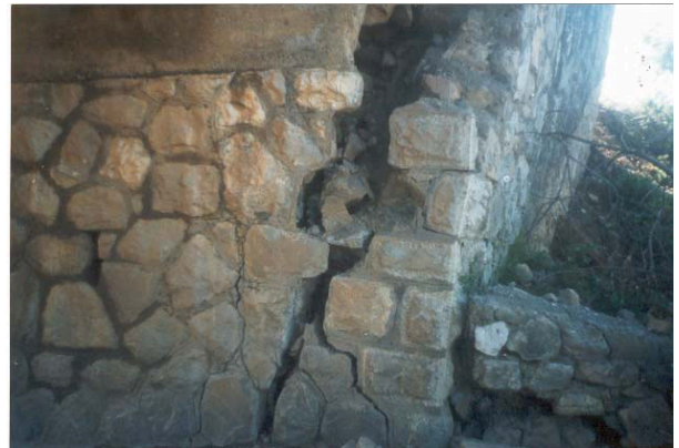
Photo nr. 6. Kallmeti bridge. It shows cracks of pillars from erosion phenomenon
