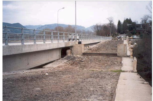
Photo nr. 2. Peshkatari bridge. It's looking to south, and shows, the new bridge and the destroyed bridge (right side) which is sunken 1.98 m compared with the new bridge.
