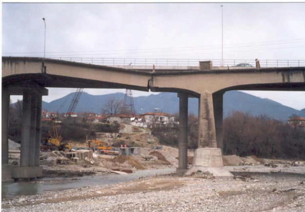
Photo nr. 1. Peshkatari bridge. It's looking to east, and shows, cracks, destroyed beam and a sinking of pier.
