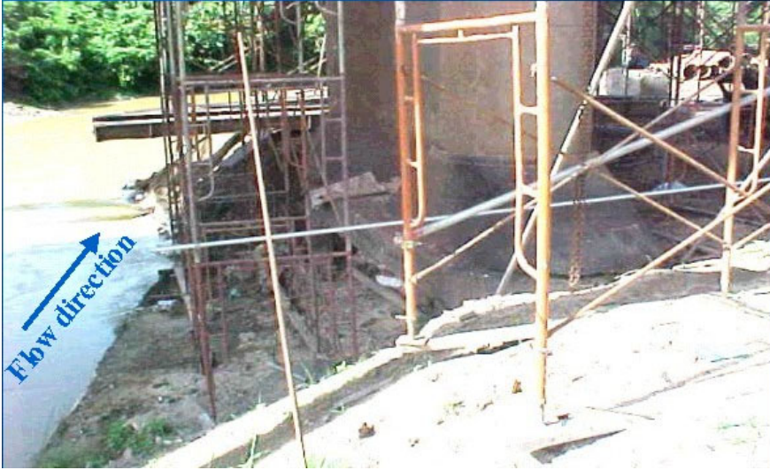
Fig. 1. Abutment scour at Muda River in Jediang, Malaysia (Photo courtesy of Shanker Kumar Sinnakaundan, River Engineering and Urban Drainage Research Center, Malaysia)
