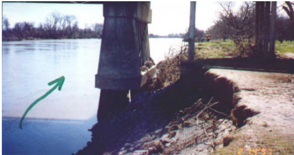
Figure 4: Scour caused by the floods of 1996/97 at pier no. 107
