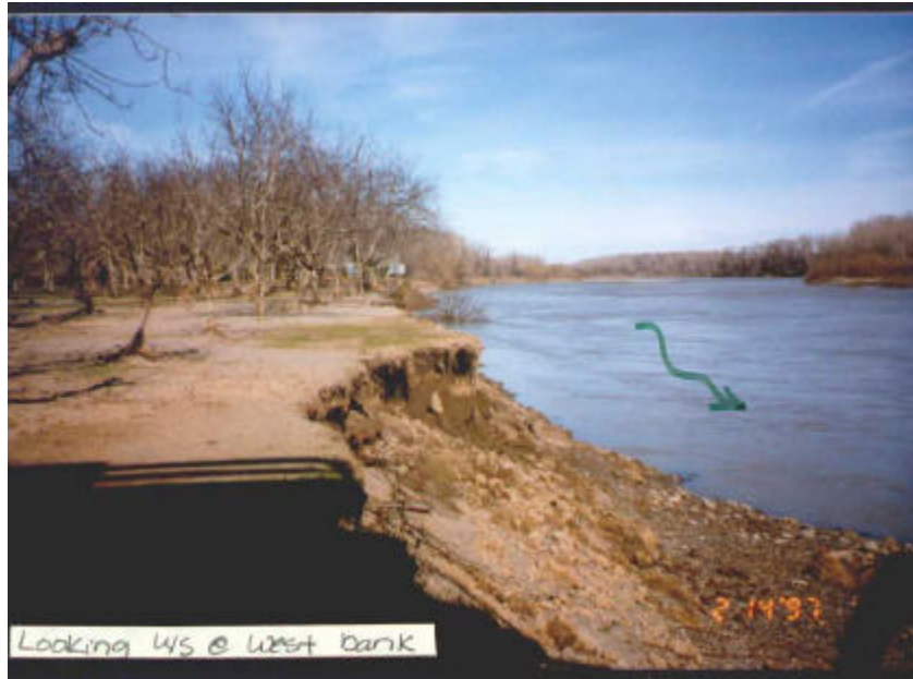
Figure 3: Erosion caused by the 1996/97 floods on the west bank
