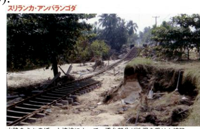
Fig.4 Damage caused by Indian Ocean Tsunami in 2004 Sumatra Earthquake. Ambarangoda, Sri Lanka Railway where bridge abutments were affected by scouring due to tsunami runup in water channel (photograph courtesy of Kyoto University Disaster Prevention Research Institute (DPRI-KU)).
